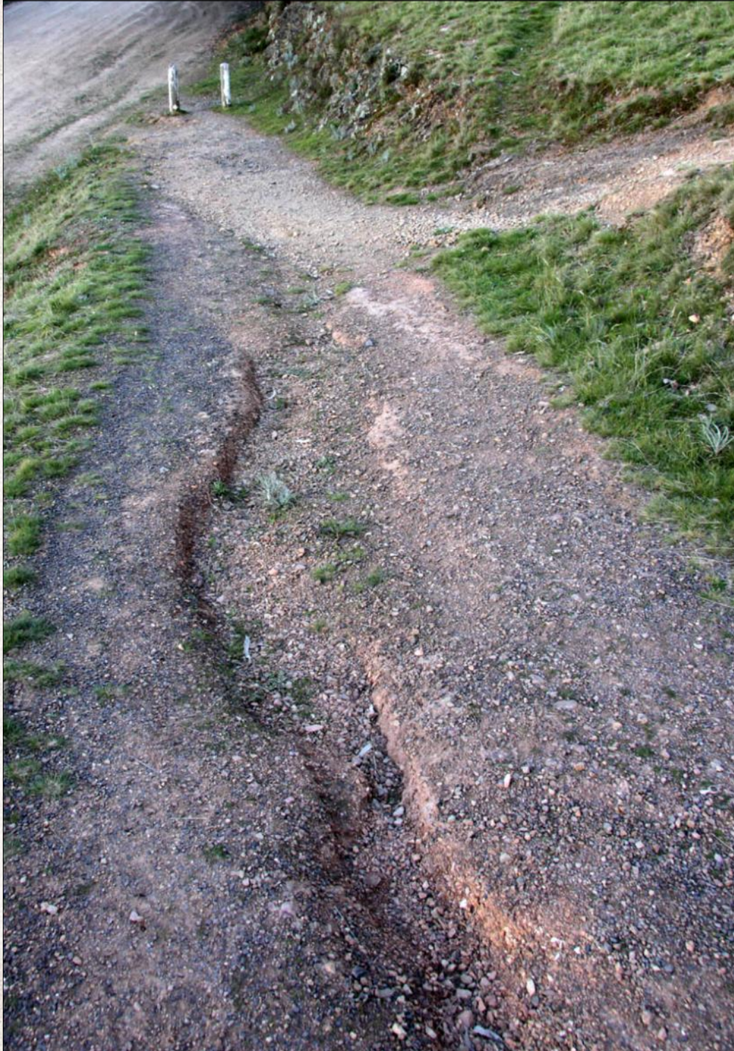
Uneven pathway in 2015 and evident from 2009–18
