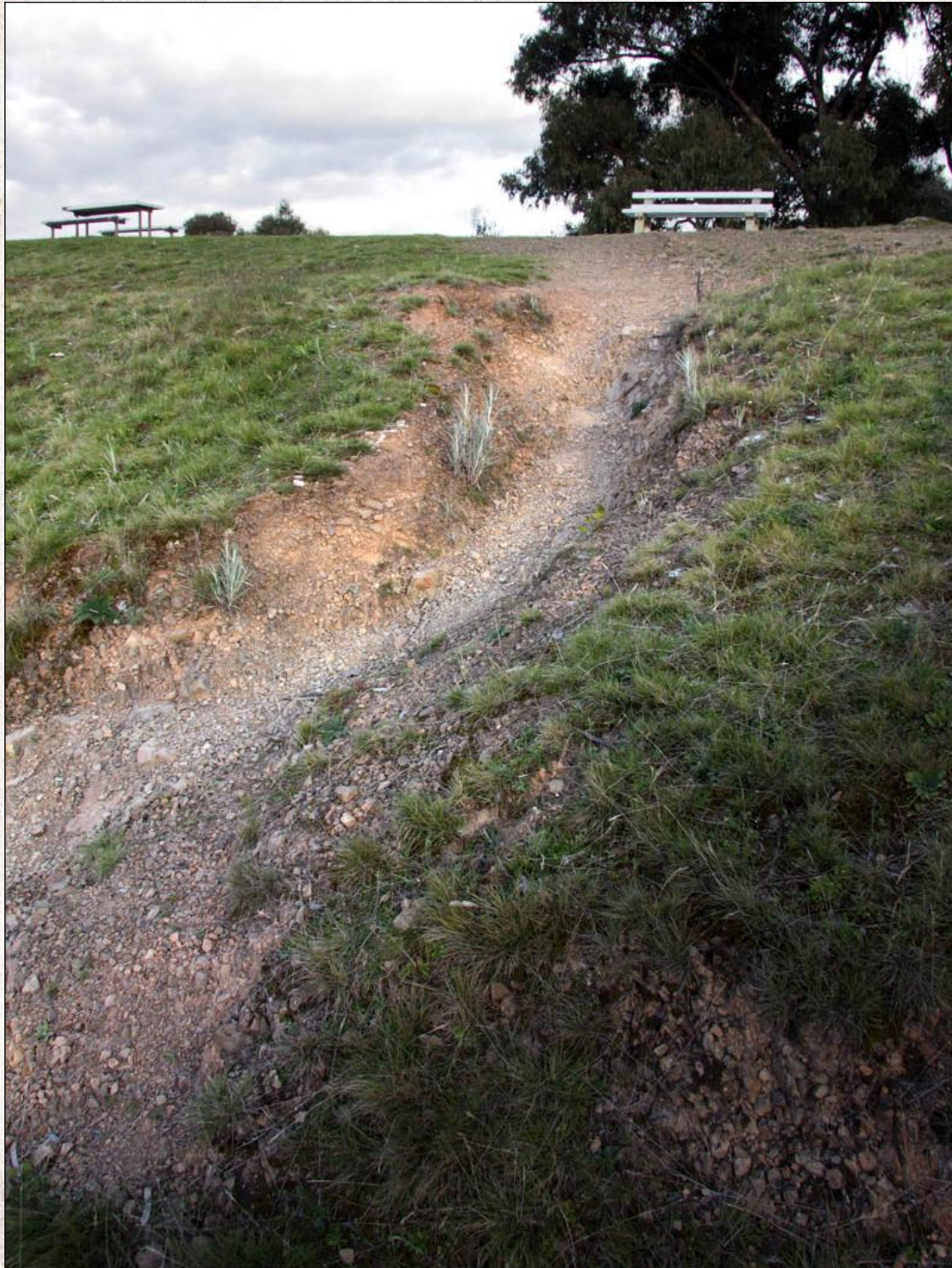
Uneven pathway in 2015 and evident from 2009–18
