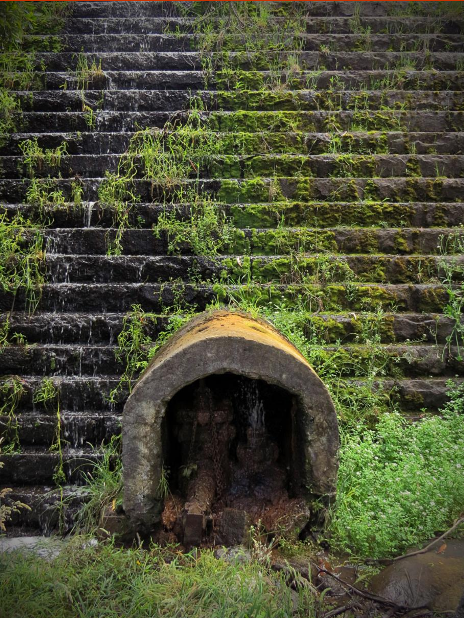
The leaking attachment where the pipe to Seymour township was once attached
