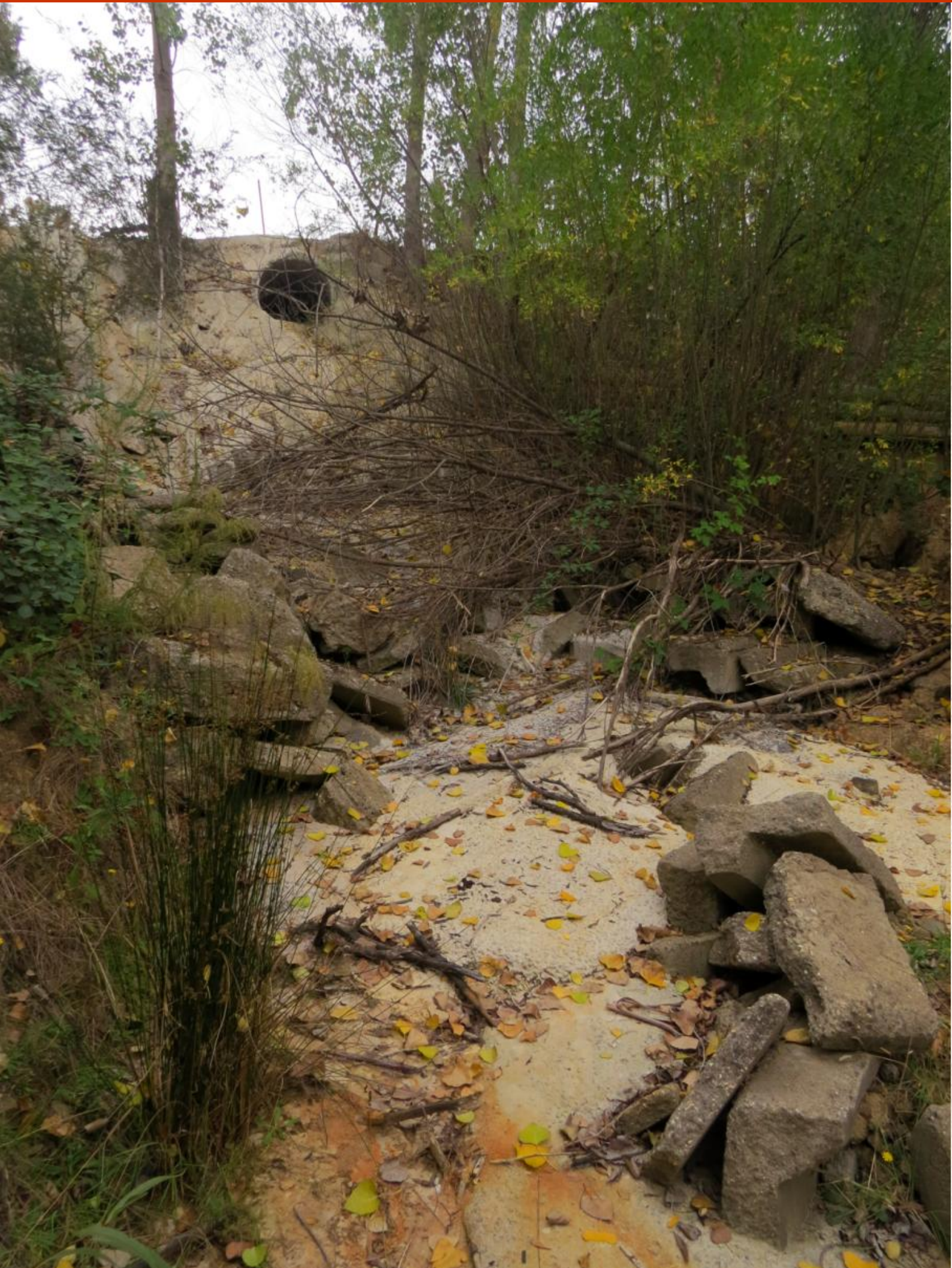
Concrete dumped off the roadway
