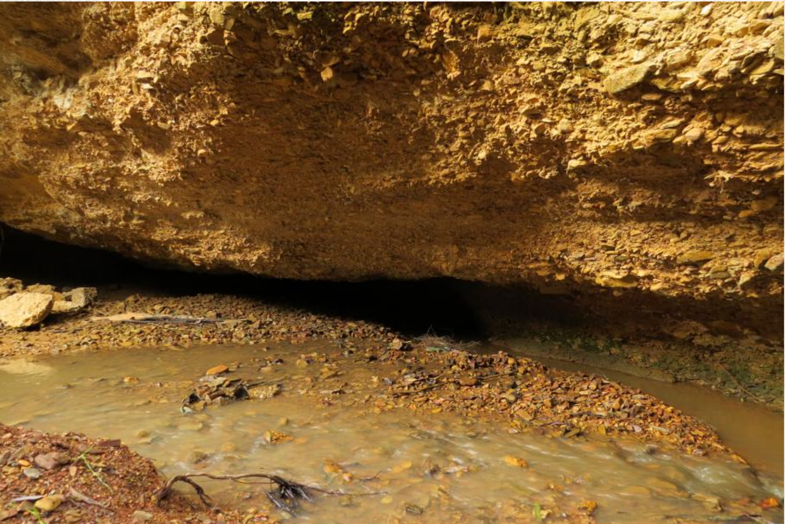
The first sign of the high banks, where a recent collapse was evident
